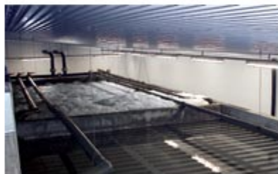
Our multi-step fluidised fixed UNI Bio Filter technology provides a completely
